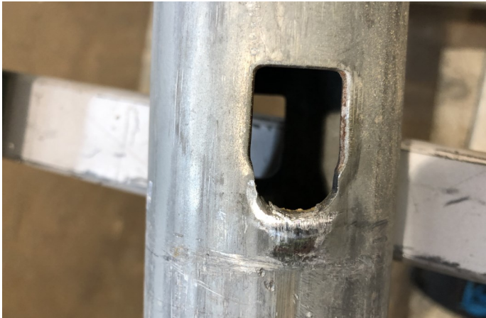
Hole at inner tube widened
